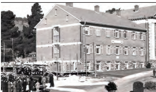
↑ Laying Foundation Stone for Ranson Mortlock Laboratory, May 1937, WARI Photo Collection, UHHP
